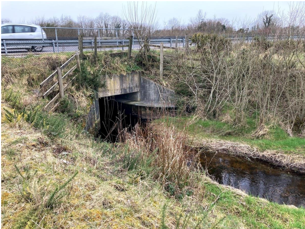
Figure 6 Existing Culvert on Ballymacahill River under the M81 Motorway - looking at the inlet face
